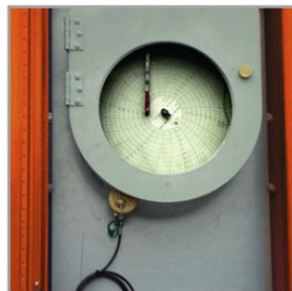
Recording instrument for tension meter
